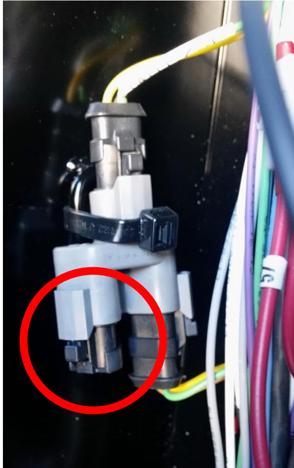
Example CAN termination (circled) can be removed when the switch on the EDT is terminated
