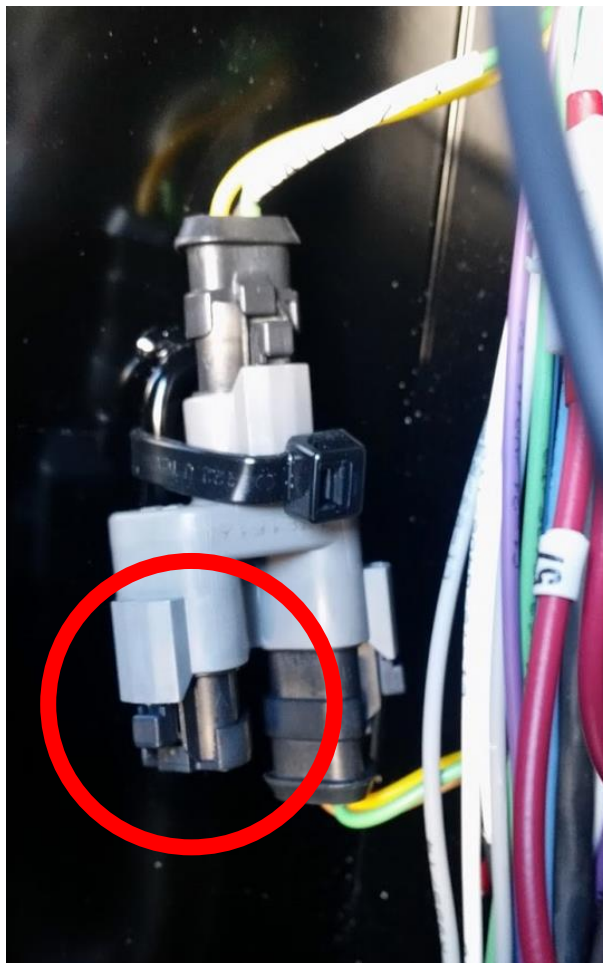
Figure 1. Example CAN termination (circled) can be removed when the switch on the EDR is terminated
